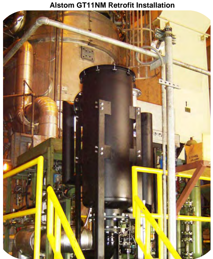
After (Clean air discharge)
