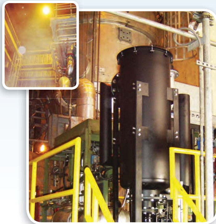
Alstom GT11NM Gas Turbine Inset: Hazardous Oil Mist Emissions from Previous Electrostatic Precipitator. After: Clean and Safe Work Environment with a Solberg Oil Mist Eliminator.
